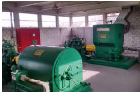
◀ BP Pipelines' Jackson Station for the River Rouge Pipeline.
